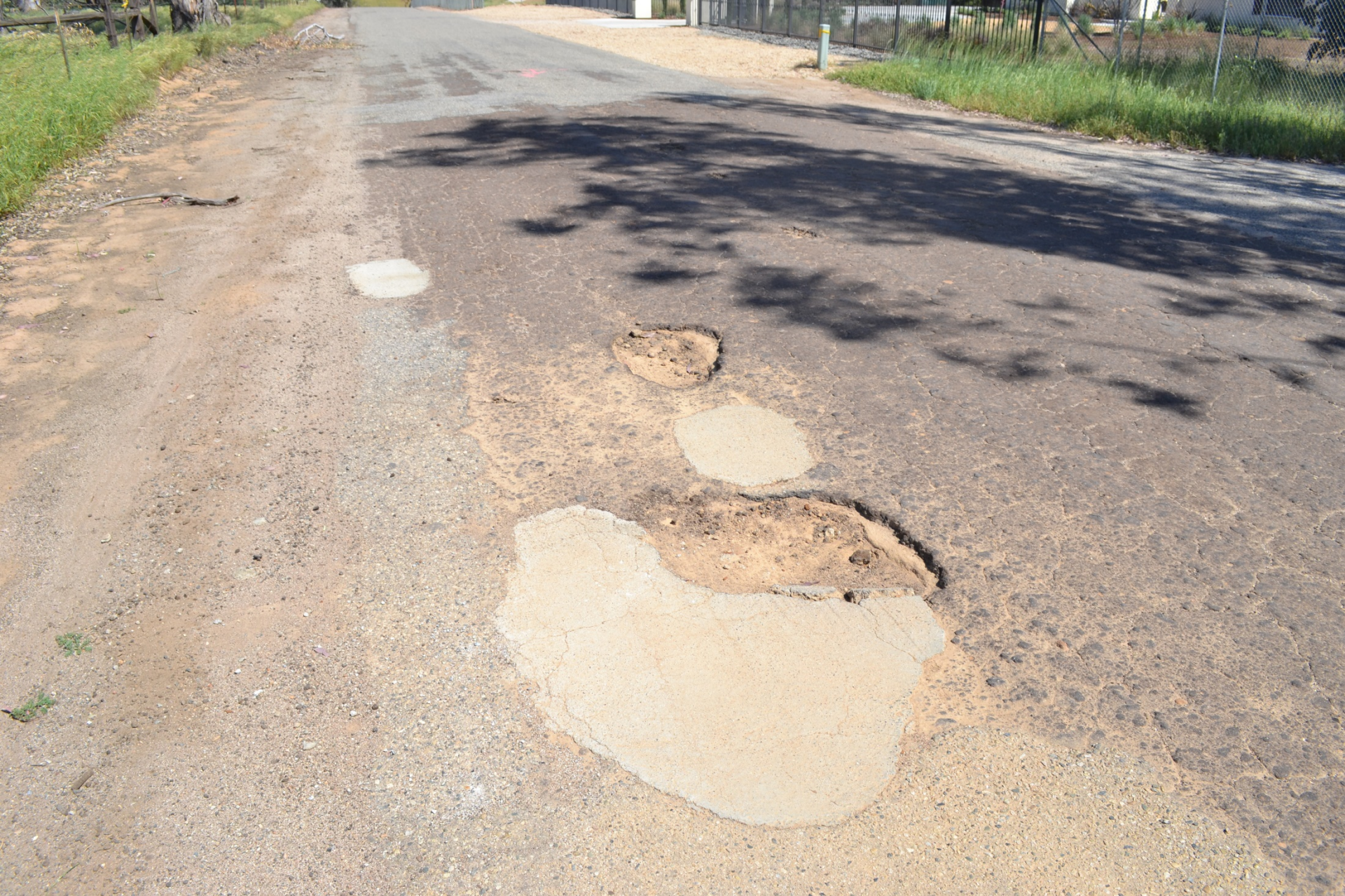
Pavement condition in front of the recent variance locations
