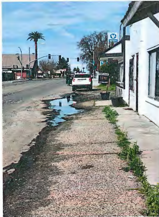
Figure 12: East side of Elm Ave facing north from just south of Lincoln Ave.
