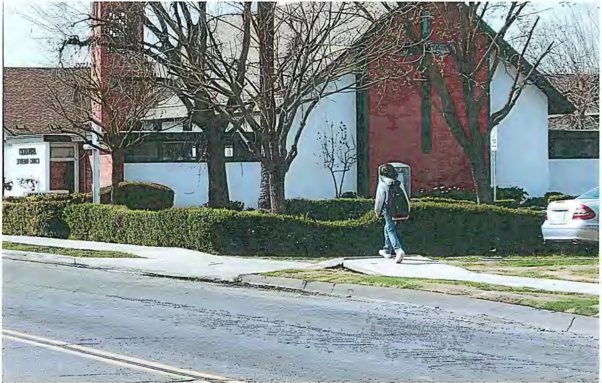
Figure 1: Student walking on buckled sidewalk on north side of Lincoln Ave near elementary school.
