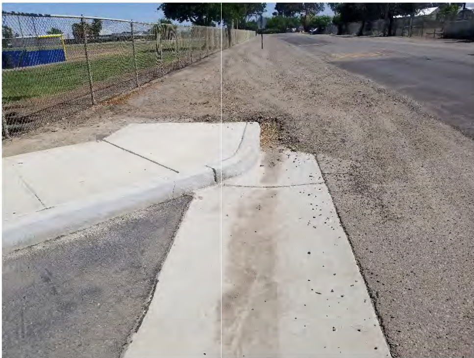
Inadequate Sidewalk near Tranquillity High School, corner of Daniels & Randolph
