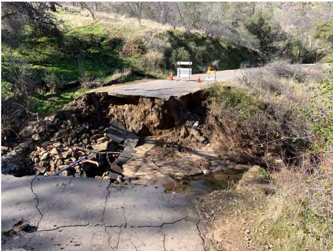
Washout due to storms on Italian Bar Road in eastern Fresno County.
