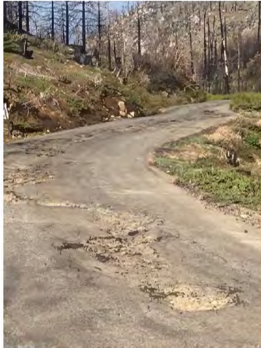
Storm damage on Hintington Lake Road in eastern Fresno County.
