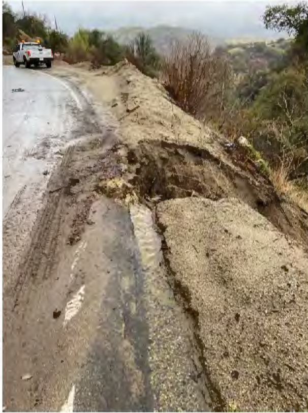
Flood damage on Dunlap Road in eastern Fresno County.
