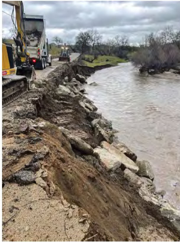
Washout due to flooding on Old Millerton Road in eastern Fresno County.
