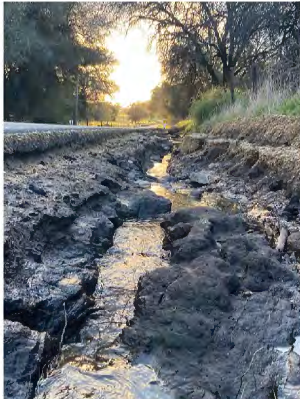
Flood damage on Ruth Hill Road in eastern Fresno County.
