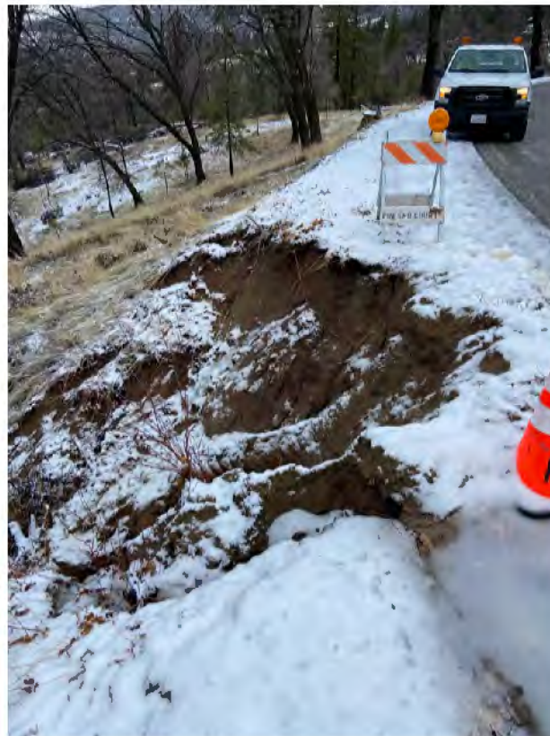
Storm damage on Hogback Road in eastern Fresno County.
