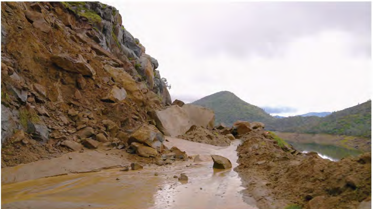
Mudslide on Trimmer Springs Road in eastern Fresno County.
